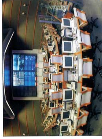
The launch control room during commissioning.
