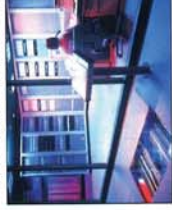
The central control room.
