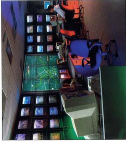
The MITSC Control Room in Detroit, Michigan, uses a videowall for both surveillance video and graphics.
