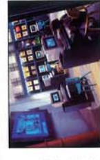
Electrosonic videowall with workstation digitiser installed in Scholastic Inc's NYC marketing facility.
