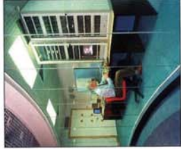
The headend room is part of the tour at HALO 2.
